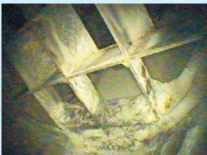
Ablagerung in Filterelement
